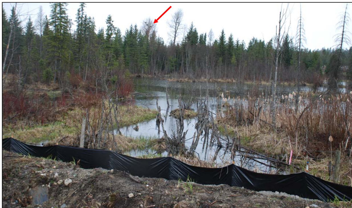
Highway 3 road re-alignment encroaching onto the wetland where Jaffray Ranch herons feed and nest.
