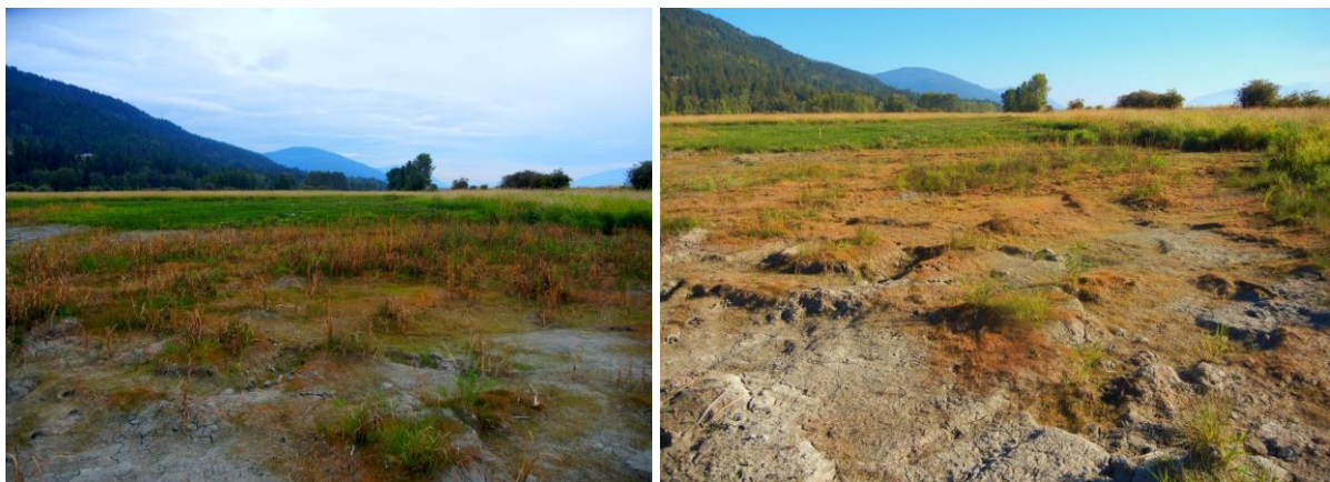
Figure 14. Cattail removal project images (clockwise from top left): Google Earth (GE) image of 6 newly constructed wetlands completed in December 2016; GE image of cattail removal treatment area in OGCS-2; treatment area before work began; treatment area when work was completed. Images 2-4 taken from Morrison, 2017.
