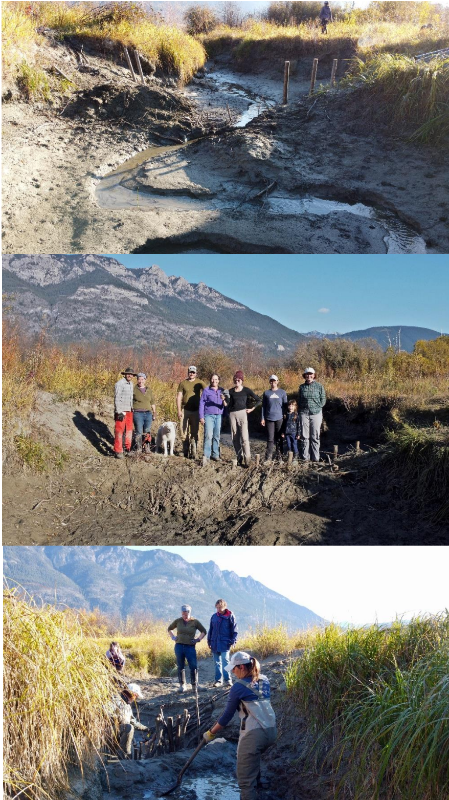
Figure 5.3. Building an artificial beaver dam at Site 38; the middle picture shows one of the completed dams.
